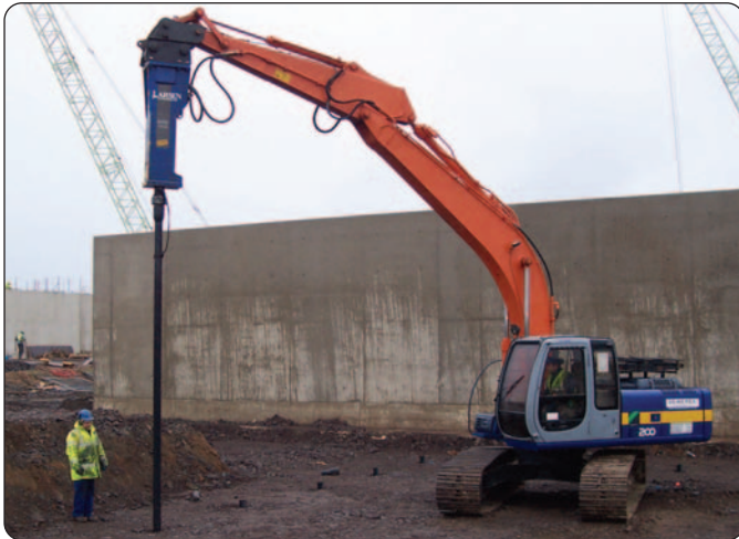
Waste Water Treatment Works
